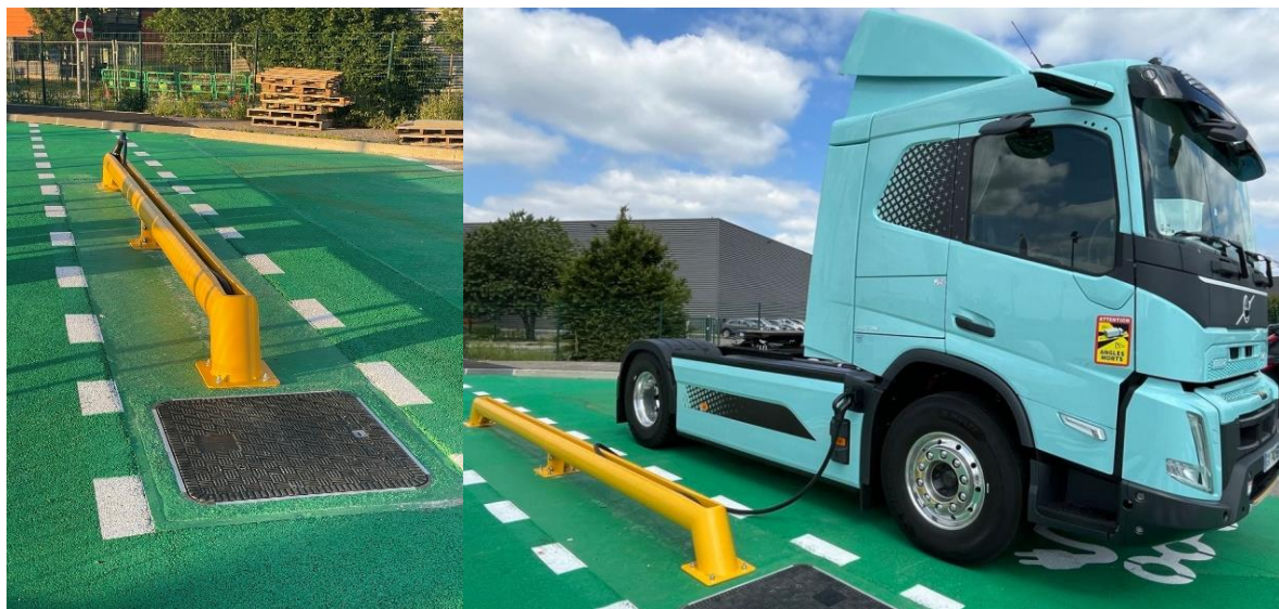
Figure 27 A space effective installation of chargers. This is made by Proviridis utilising a Kempower solution. Image from Kempower.
