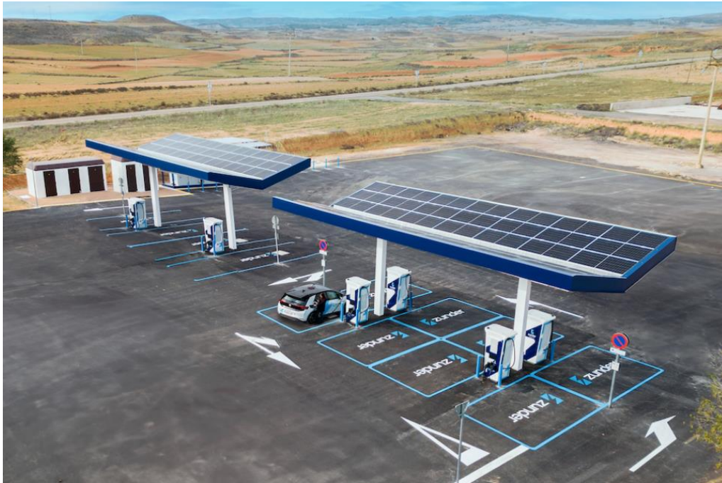
Figure 29 Zunder charging station, Cetina, Spain. Image from Zunder.
