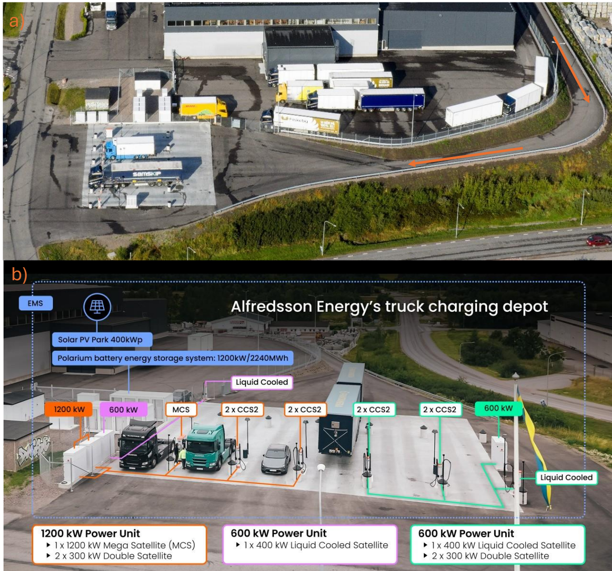
Figure 34 Alfredsson Energy, a MCS charging station in Norrköping, Sweden. a) To get a straight angle when entering the charging points even with a HCT (34,5 m), the trucks drive around the terminal house (outside the fenced area). Image from Alfredsson Energy. b) The charging point setup. Image from Kempower.
