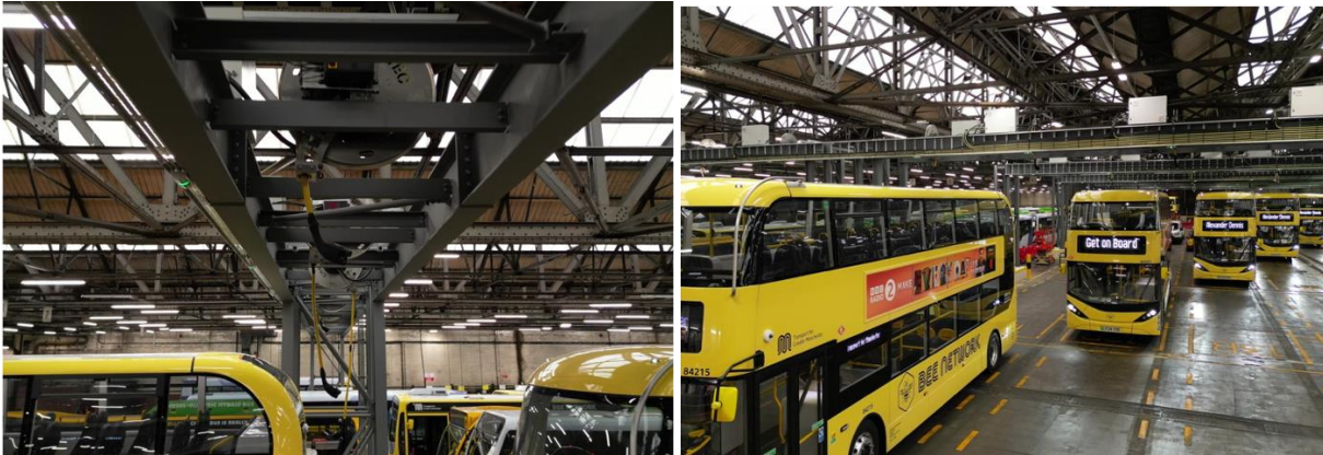
Figure 26 Overhead gate charging at the Walshaw Street bus Depot in Oldham, used as a solution to adapt to the current layout of the parking bays for buses. Image from Janus Architecture.
